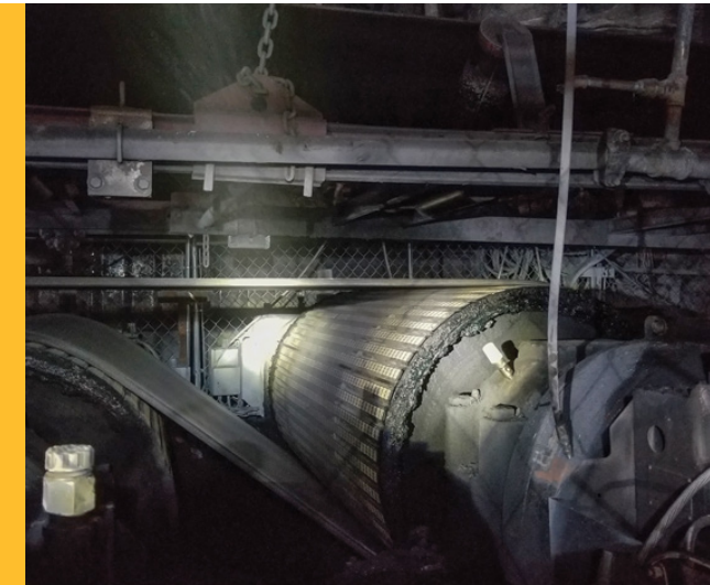
A critical belt conveyor used for transporting material from the underground mine to the surface.
