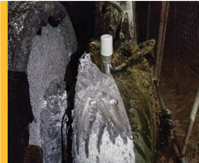
An OPTIFY Performance Sensor installed on a mounted bearing, attached to a belt conveyor inside the underground mine.
