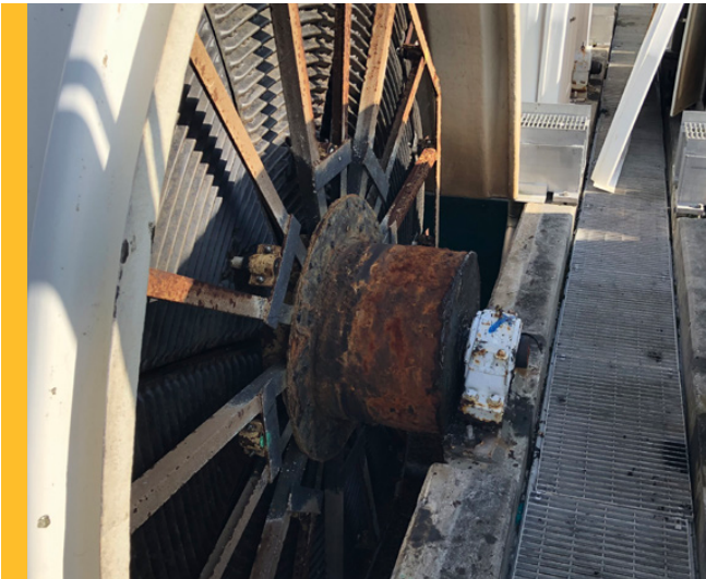
Because RBCs operate so slowly, equipment failure often isn't found until it's too late. The failure on this RBC wasn't found until the media assembly shifted, contacting the concrete and tripping the motor.
