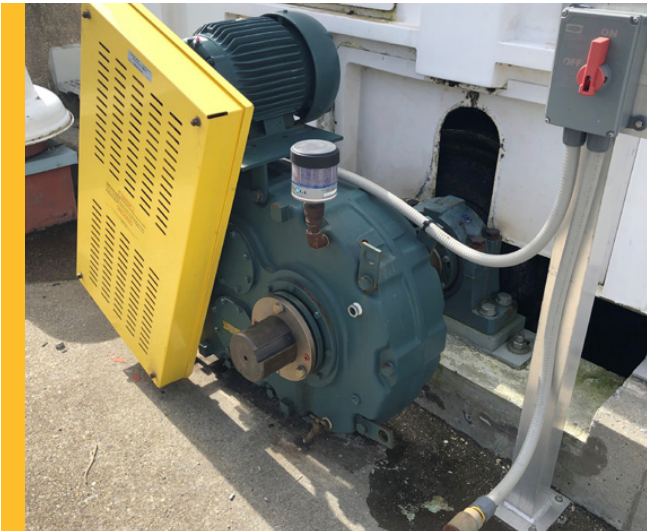
In addition to switching to Safety Mount for its superior seals and quick installation, the plant transitioned to a complete Dodge drive package with BioDisc gear reducers and desiccant breathers for enhanced reliability and valuable savings.
